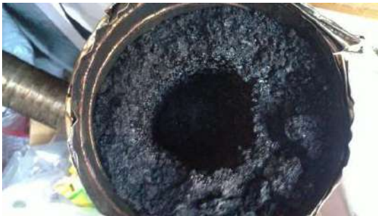
150mm chimney liner blocked with deposits
